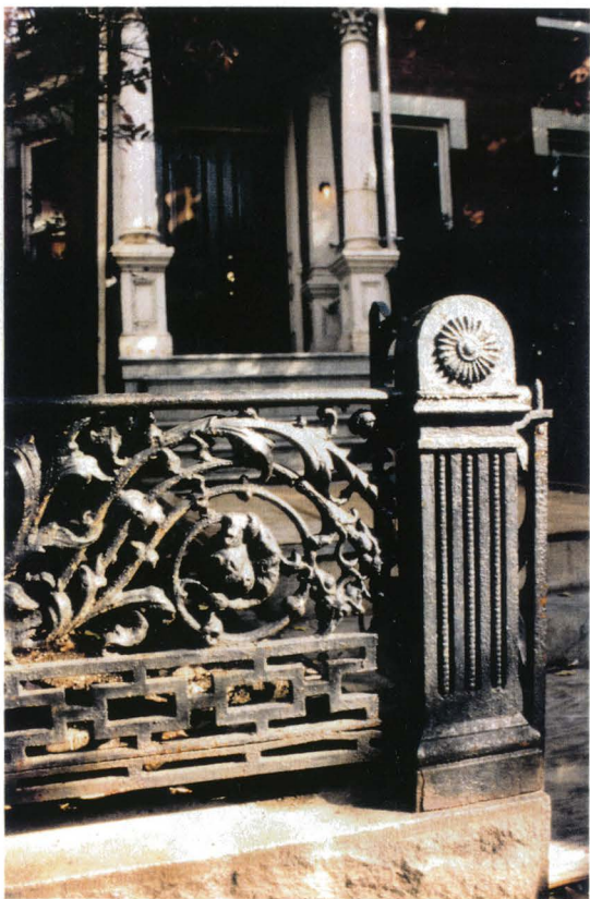
Figure 33. Cast iron fence in front of Gunn-Bird House, 820 West Franklin Street (Photo: Chris Dunham)
